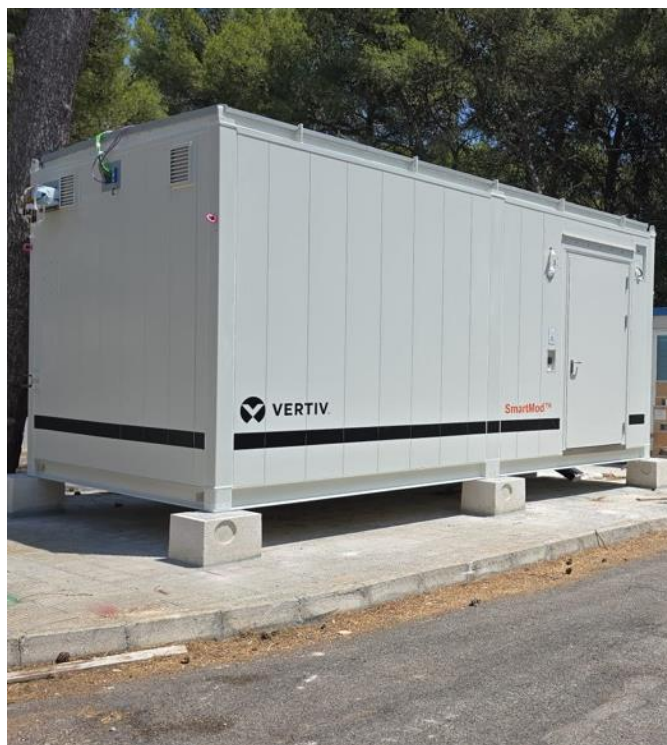
E-RIHS Cloud Data Center – Lecce- Catania-Napoli
